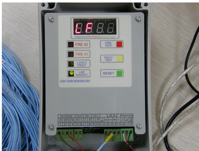
Figure 11.2 – Power on MCU
